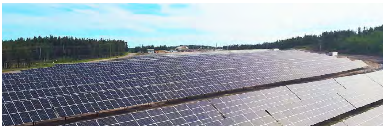
Fort Chipewyan Solar Project, Fort Chipewyan, Alberta
