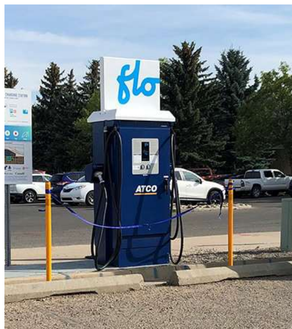
EV charging station, Lethbridge, Alberta
